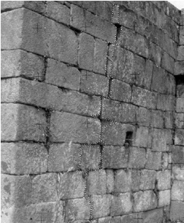
FIG. 4. Cloud of points corresponding to the crack outline.
